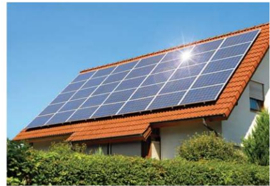
▲ Figure 12 A domestic photovoltaic panel system.
